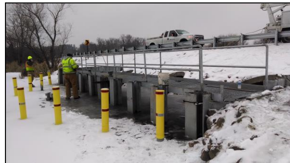
Martin Lake north inlet (completion in early 2016)
