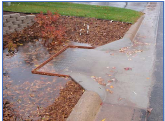
Pretreatment chamber prevents leaf litter and sediment entry into garden (Area 2).
