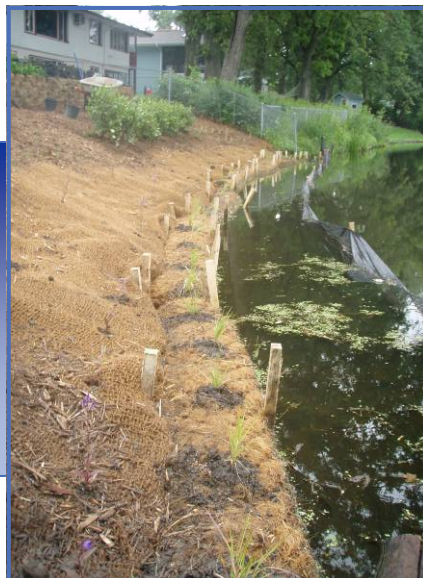
Bioengineering practices like this biolog provide water quality benefits, shoreline stability, and increased wild-life habitat.
